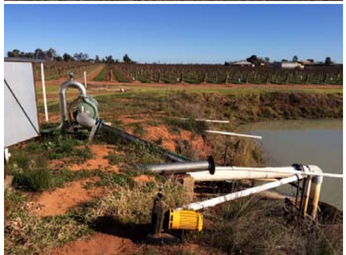
Pump station (inside shed) and the pump suction line leading into the on-farm dam.
